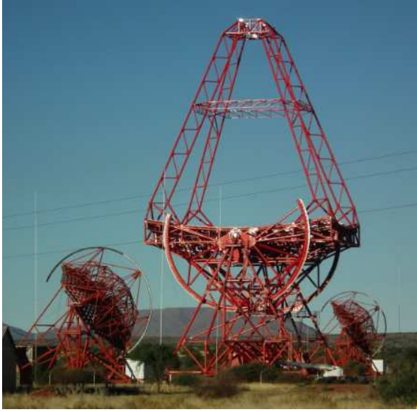
Figure 15: The steel structure for the 600 m 2 H.E.S.S. II telescope. Mirrors and camera will be installed in the first half of 2012. (Note that the H.E.S.S. II telescope is located in between the two H.E.S.S. I telescopes shown in the image, not in the foreground). Figure courtesy of the H.E.S.S. collaboration http://www.mpi-hd.mpg.de/hfm/HESS/
